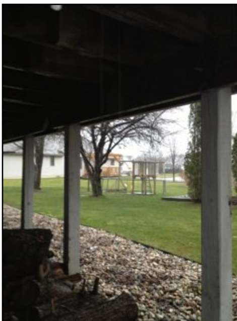
15. End support inadequate
