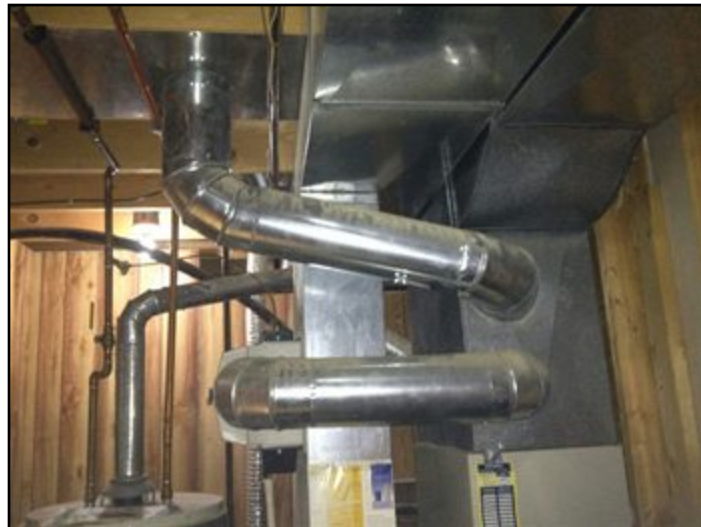
26. Ducts and registers
