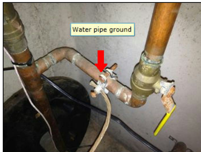
22. Copper - water pipe
