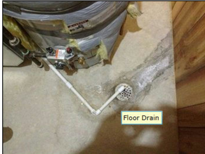
41. Near heating system
